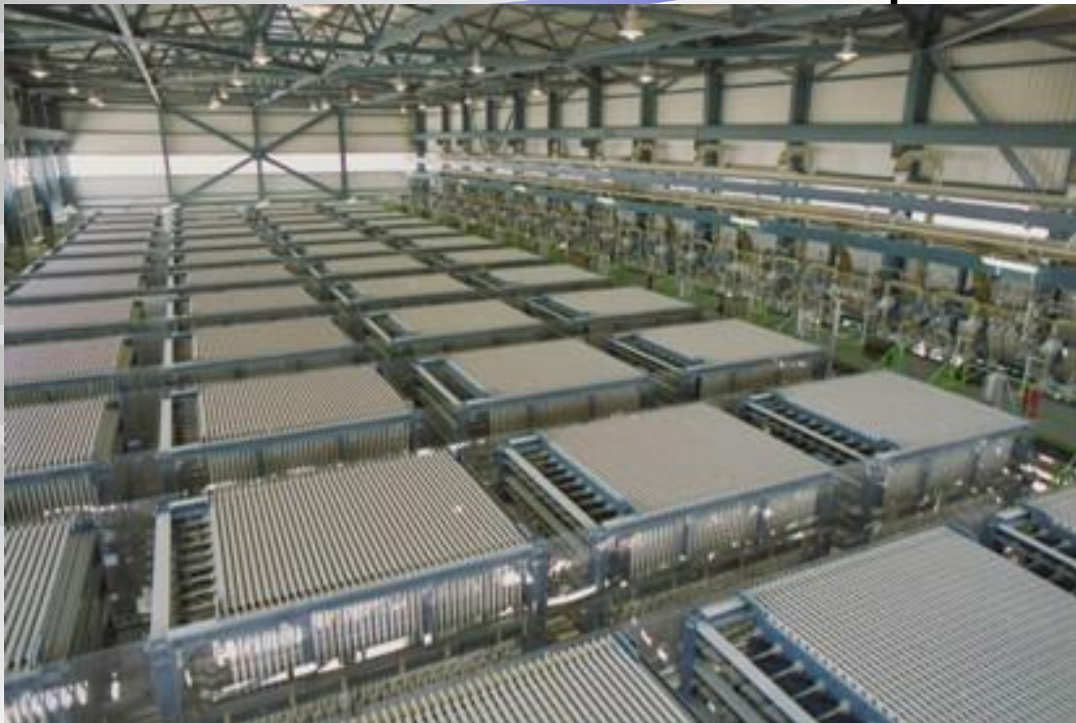
Chlor-alkali cell room with BL-2.7 membrane cells (Courtesy of Uhde GmbH).
